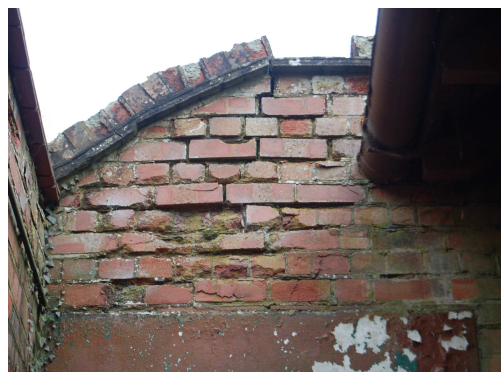
The buildings at RAF Bicester remain in poor condition whilst the Crichel Down process is concluding.
